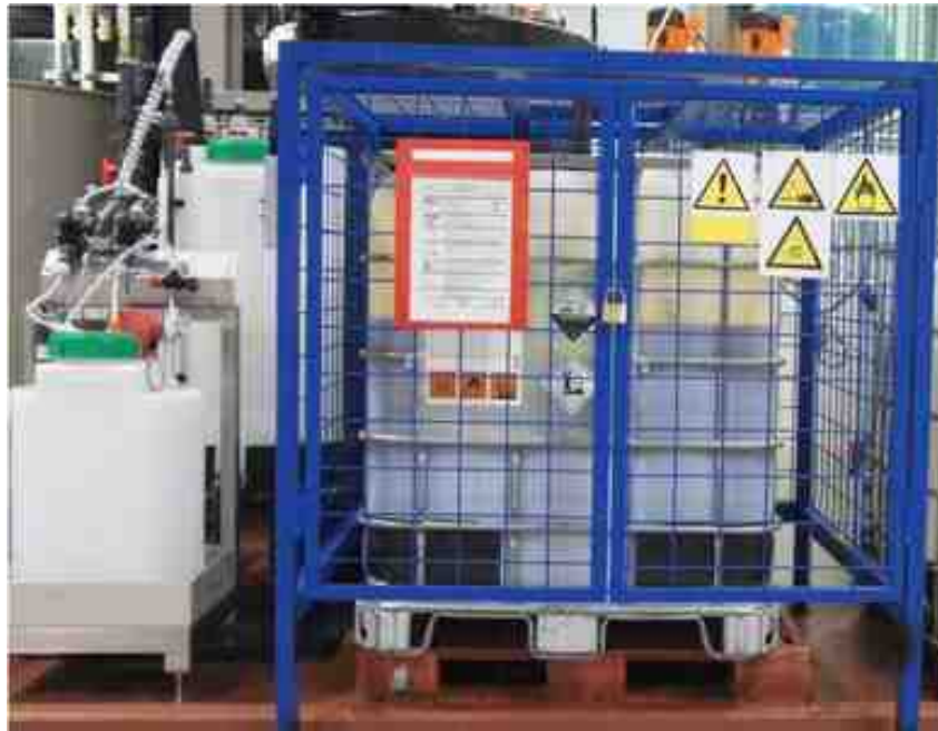
Figure 13 - Liquid hexavalent chromium additive pumping station.
