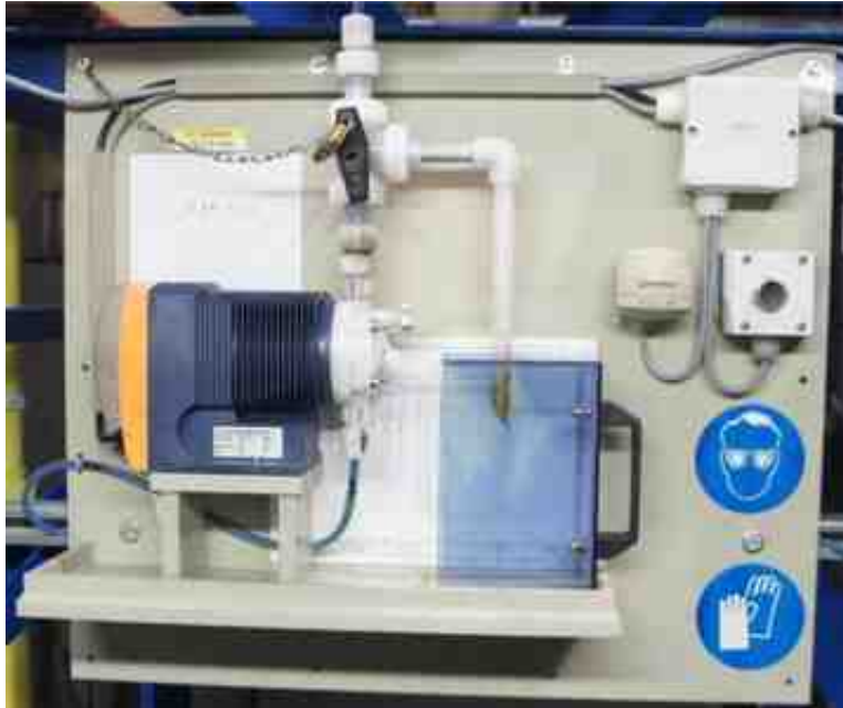
Figure 14 - Pumped sampling station.
